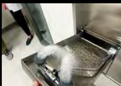
Emergency eyewash fountain in science lab.
