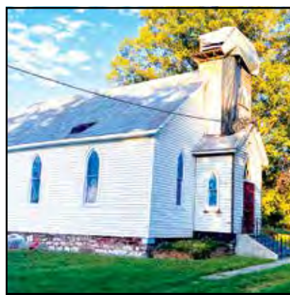
Historical Warren United Methodist Church is getting a new steeple and needs some financial help.
