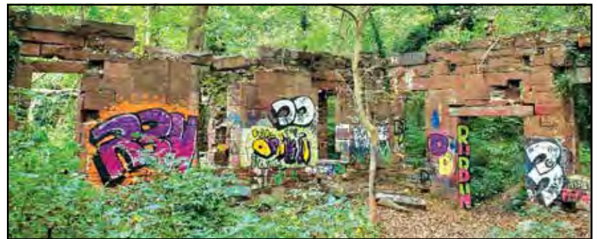
Graffiti on the Seneca Aqueduct.
