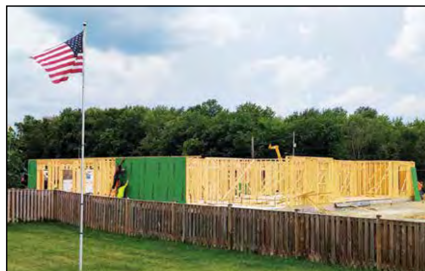
Homes for Our Troops new home now under construction in Poolesville. See the photo collage of the Kickoff Celebration on page 11.
