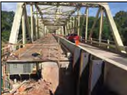
The Monocacy River Bridge project is almost finished! Get the scoop on page 8.
