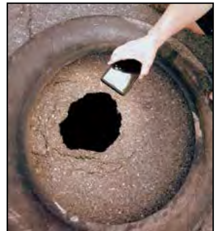
This small opening uncovered a large, cavernous space under a parking lot.
