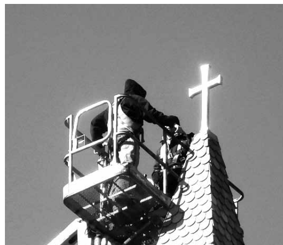
Roofing contractors complete the installation of the new cross at St. Peter's.
