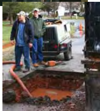
A water line broke, but this team of hard working town employees has done it all before.
