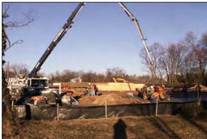
Cold weather stalled the progress on the new Poolesville town hall, but the foundation was recently poured and completed and very soon the framing will begin.
