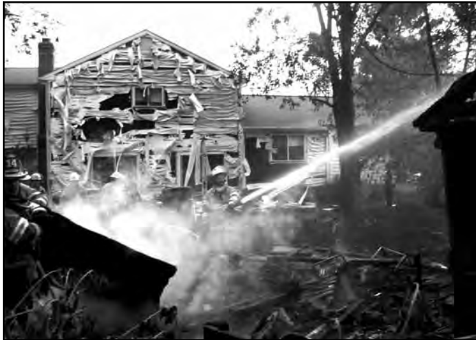
Fire from three sheds caused siding to melt on a home in the Westerly subdivision in Poolesville.
