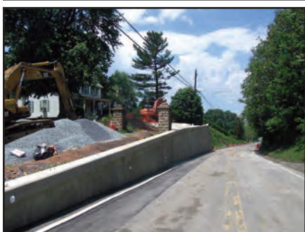
The cemetery wall is repaired, Route 28 is open, Big Woods Road returns to normal.
