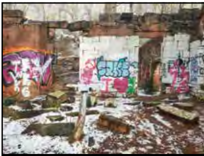
Monocacy Aqueduct vandalized.
