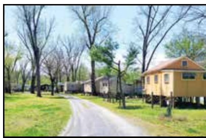
Cabins on stilts scheduled for demolition at the C&O Canal near White's Ferry.
