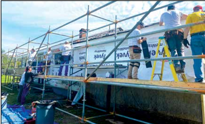
A team of over twenty volunteers replaced the siding on the Mason home and made many other repairs.
