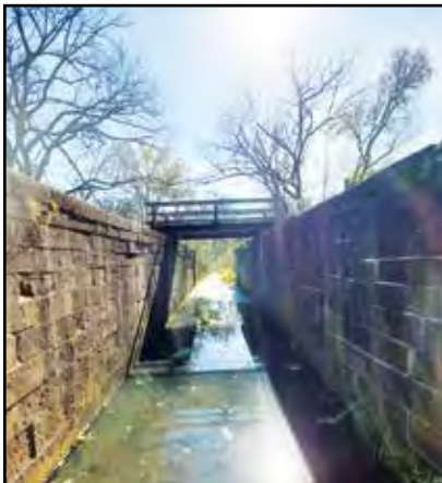
Looking through Lock 25 from the upstream end of the lock. Read more about the lock on page 10.
