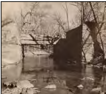
This is one of eleven aqueducts that played an important role during the Civil War. Learn more on page 12.
