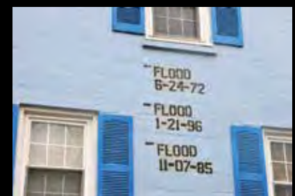
Flood marks painted on the side of the building show the height of previous floods.
