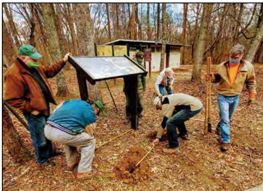
C&O Canal volunteers and a National Park Service ranger installed one of the three wayside signs at Carderock along the C&O Canal.
