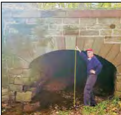
The culvert height measures seventy-eight inches. Originally, it was ten feet. Find out what happened on page 8.
