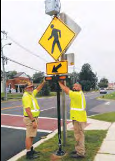
Preston King and Matt Warfield installed the new flashing crosswalk sign at Whalen Commons.
