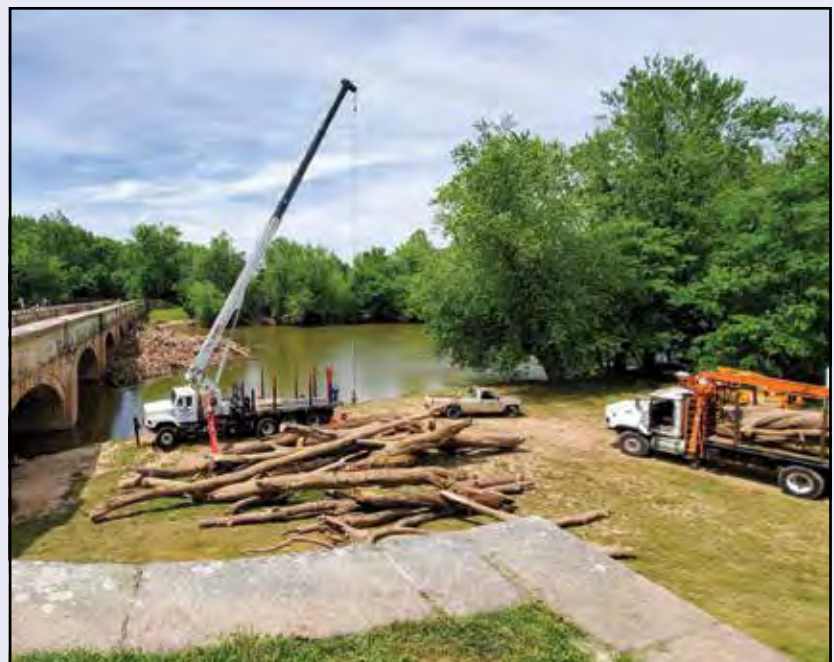
Spring floods made for a very heavy cleanup of the Monocacy Aqueduct.
