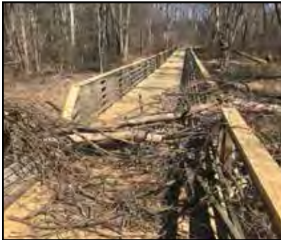
Wild and blustering winds slammed trees onto this walkway bridge between Tama I and Tama II. Read about it in Tidbits on page 5.
