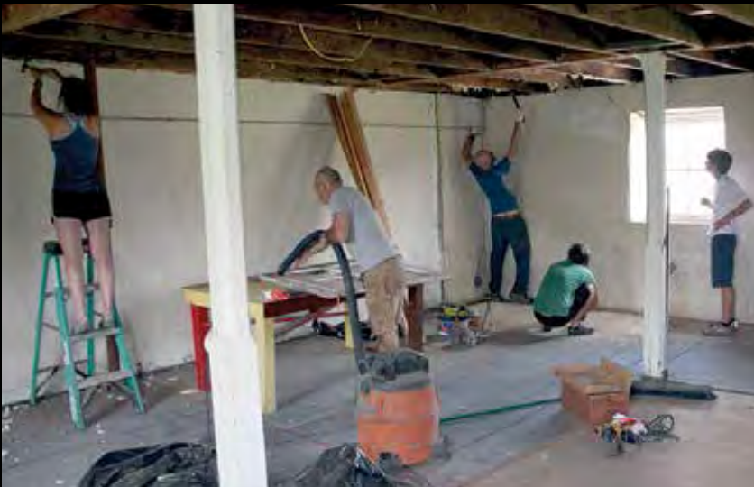
Volunteers from Calleva put up new drywall at the Friendly Thrift Shop on West Willard Road in Poolesville.
