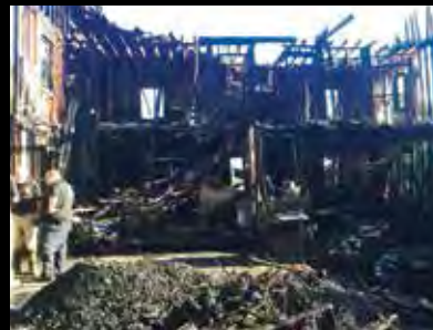
Brian Jamison's home in Point of Rocks was a total loss after a fire started by an electrical problem.
