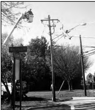
What's left of a transformer dangles dangerously over Fisher Avenue, causing early morning traffic problems in Poolesville.
