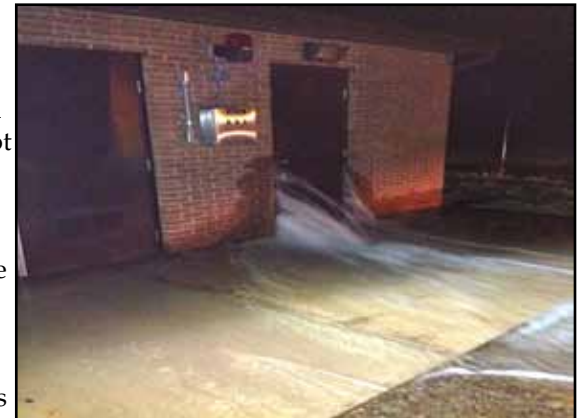
A broken coupling flooded well house in Poolesville.
