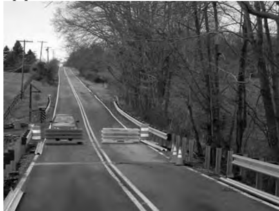
The damaged section of Barnesville Road that necessitated its closing.
