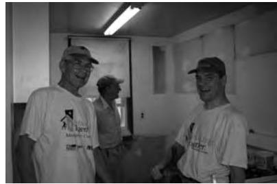
Ray Hoewing, Elmer Frohlich and Link Hoewing, get ready to install some kitchen cabinets.
