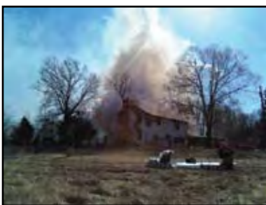
Bad news for an old house in Barnesville. See Local News on Page 7. (Photograph by Kimberly Kempa.)
