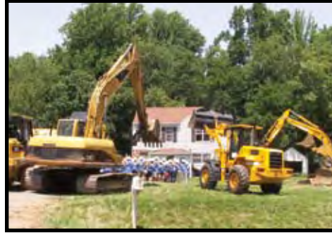
The crew and the demolition team surrounded the house just prior to starting the job.
