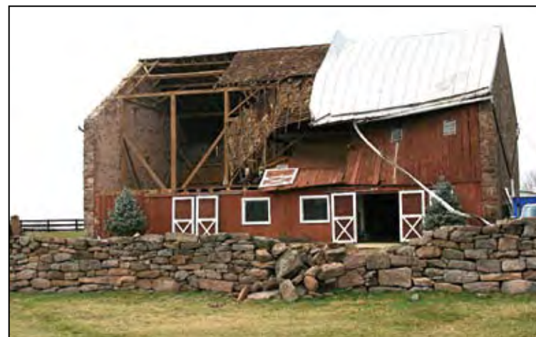
A barn in the Dickerson area with its roof blown off.
