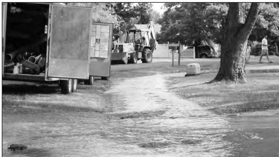
The broken water main on Hempstone Avenue.
