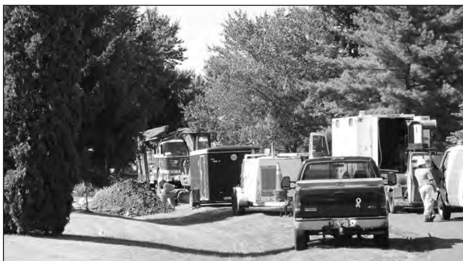
Gas main break on Soper Street.
