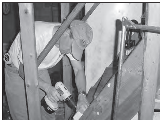
Poolesville commissioner Link Hoewing, an accomplished carpenter, is a regular volunteer for Rebuilding Together.
