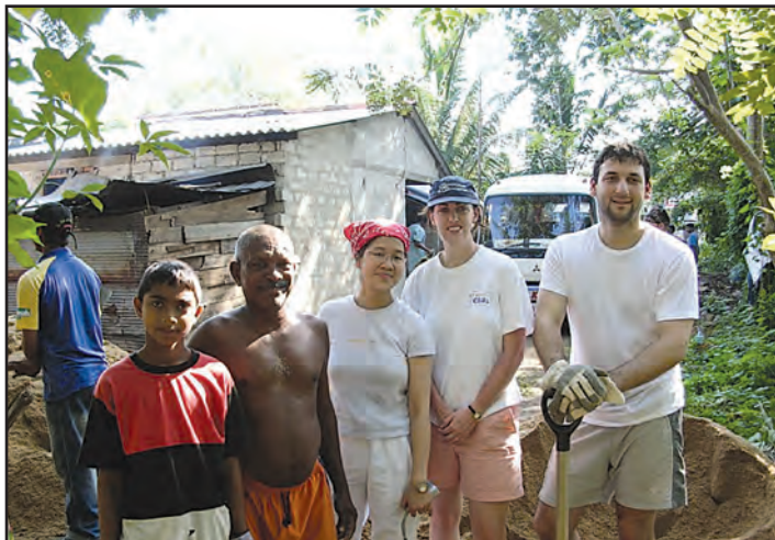
Villagers and Habitatat for Humanity volunteers rebuild. The author, Christine O'Connell, is second from the right.
